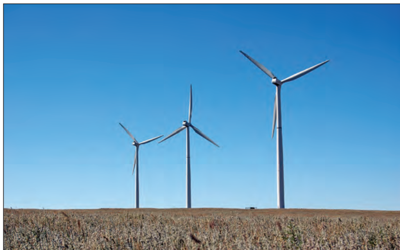
Xcel Energy set a new record Oct. 2 when wind energy supplied 54.3 percent of the power delivered to Colorado customers for the entire day.
